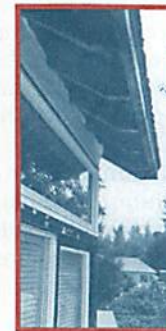
Open eaves, vents not screened (6 pts)
